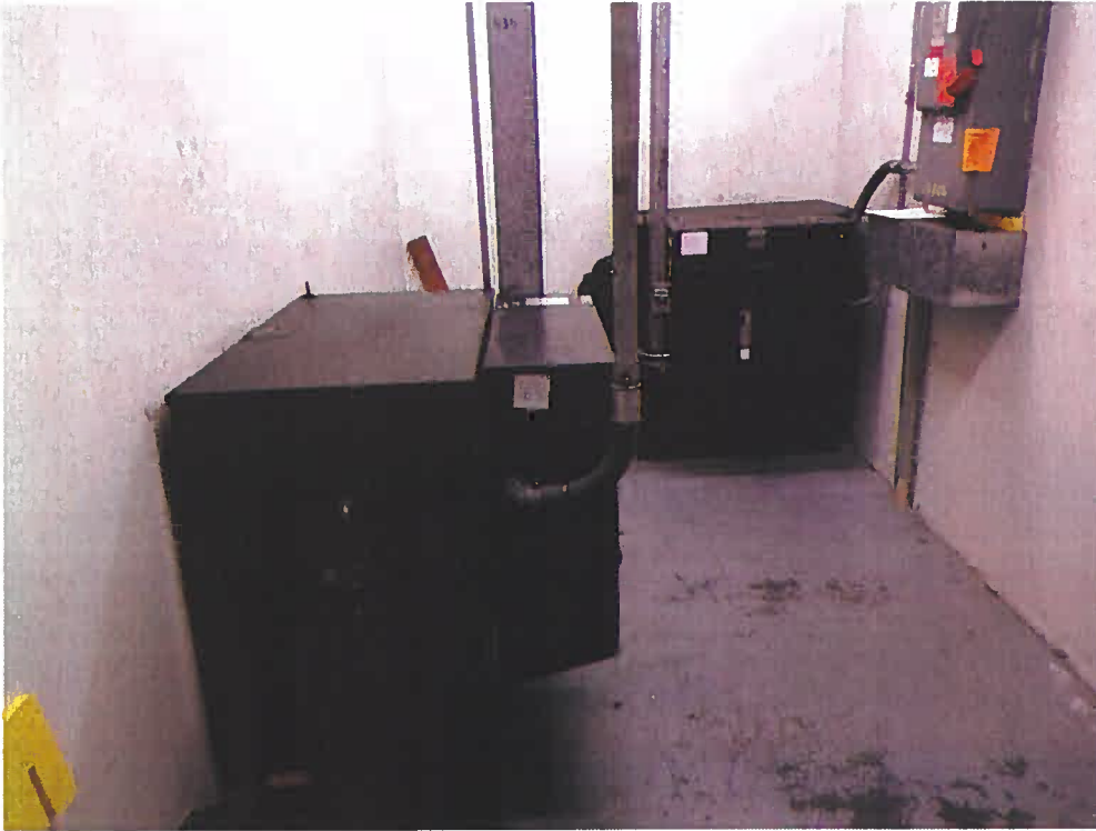
Exhibit O: Elevator Hydraulic Pumps
