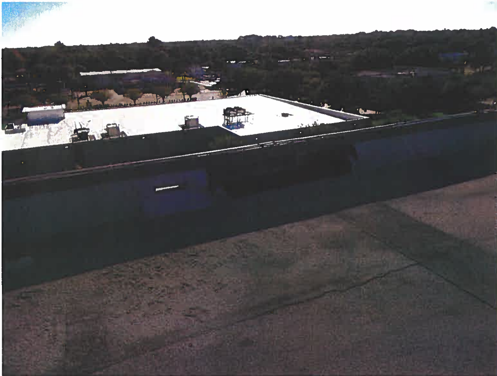
Exhibit H: Damaged Parapet Flashing
