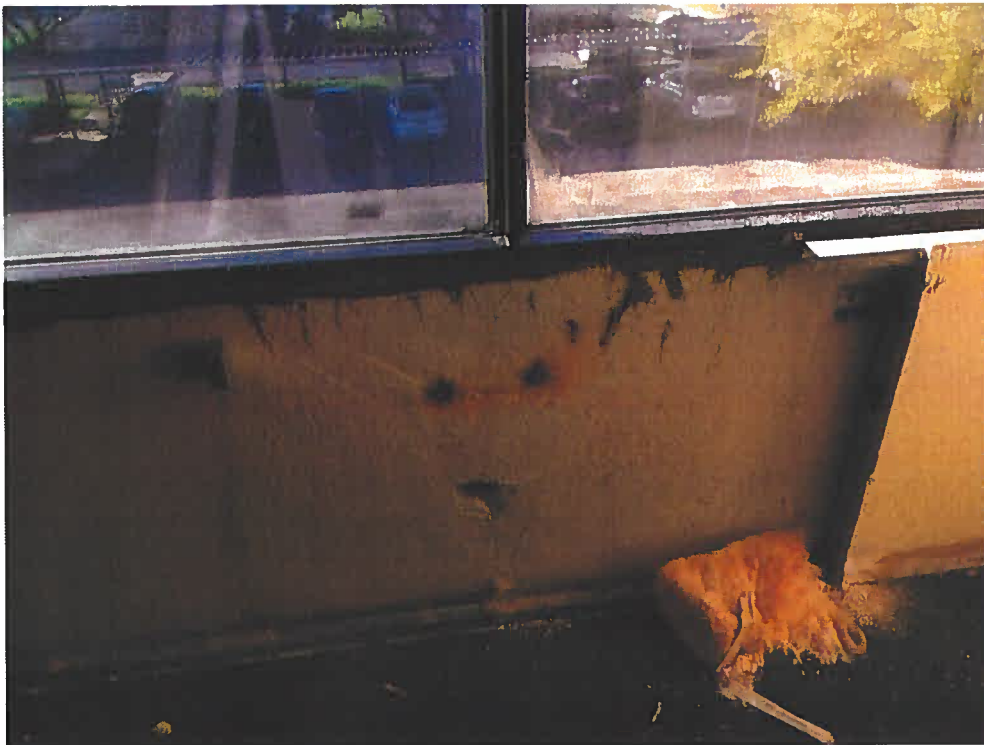
Exhibit R: Typical Example of Minor Demolition at Locations of Water Infiltration
