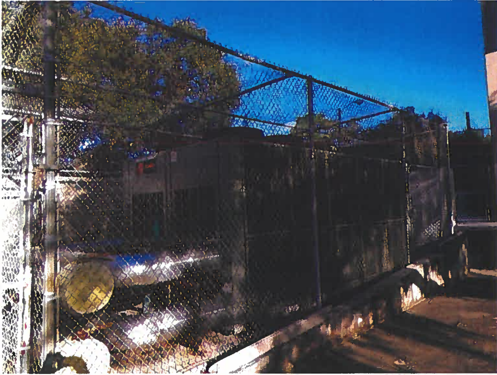
Exhibit E: Chiller Yard
