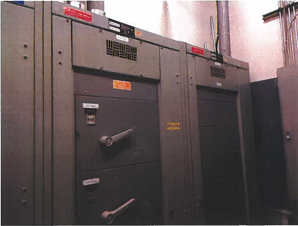
Exhibit M: Main Switch Gear
