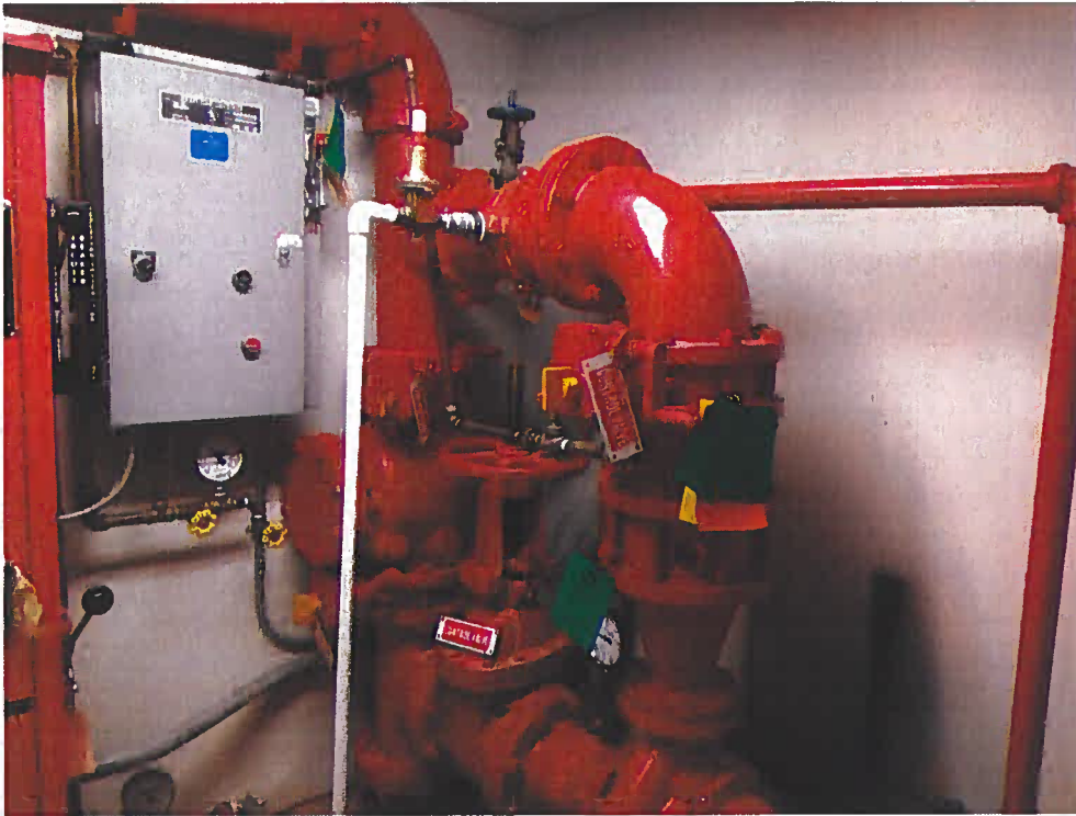
Exhibit K: Fire Sprinkler Riser in Stairwell
