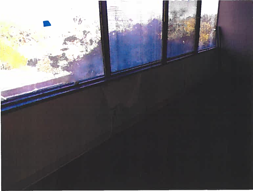
Exhibit Q: Typical Example of Vinyl Wall Covering Delamination at Point of Water Infiltration
